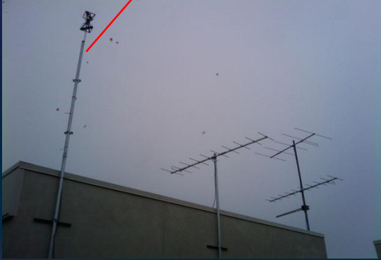
WS Antenna on Bldg 42
