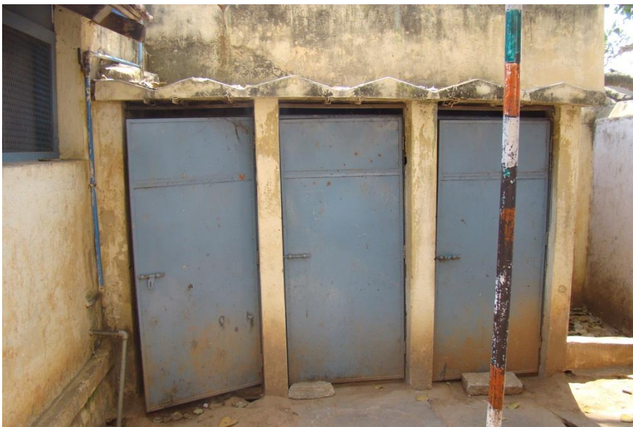
Figure 9. A sample of poorly maintained urban school toilets
