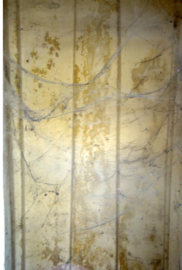
Figure 11. Upper half of toilet
