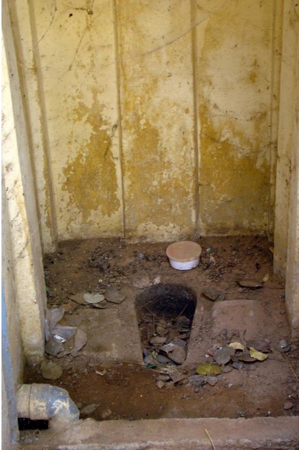
Figure 10. A blocked and dirty toilet
