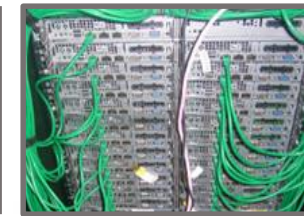
IT Equipment (servers, network)
